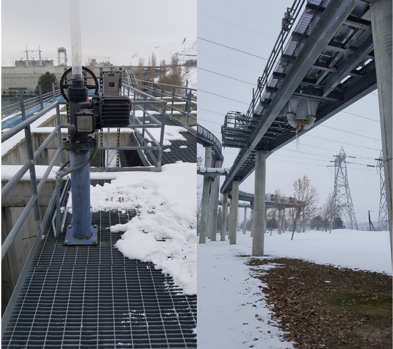
(PDS, adult fish drain valve, actuator, and switch gate circulating valve)
